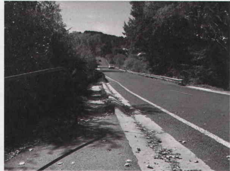
Current exit from Lake Daylesford on to Bleakely Street. Pedestrians are directed almost immediately on to the roadway.
