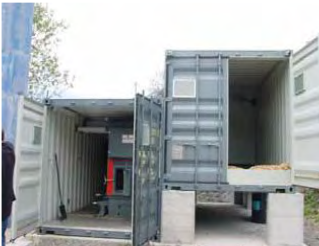
Figure 2 - Containerised Small boiler unit
