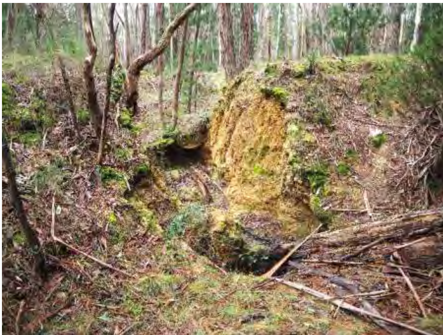
Photograph 14 Eatons race, Breached embankment at small dam
