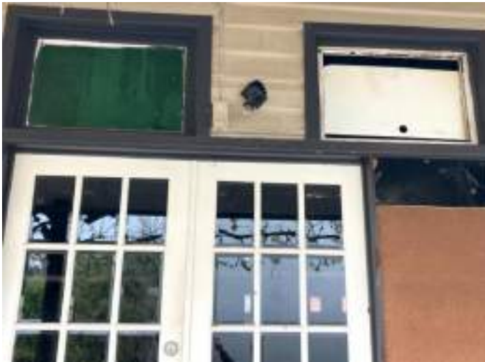
Figure 6 Introduced double doors, with original fanlights of two separate front entry points remaining on facade
