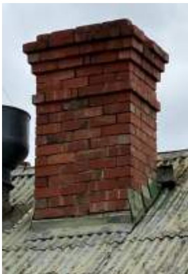
Figure 7 One of the two brick chimneys. Note the dimensions and scale of the chimney is more typical of a Victorian chimney than Edwardian
