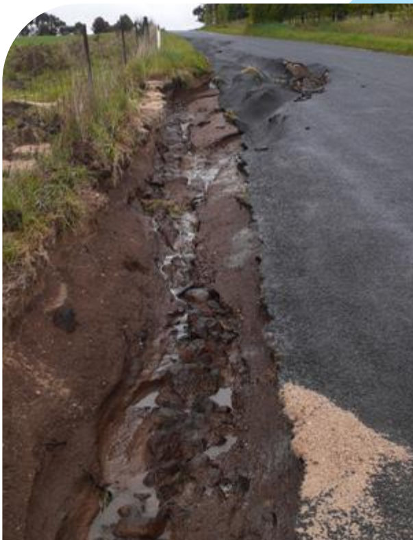
Before and after. Storm damage along Learmonth Road at Clunes in October and December 2022.
