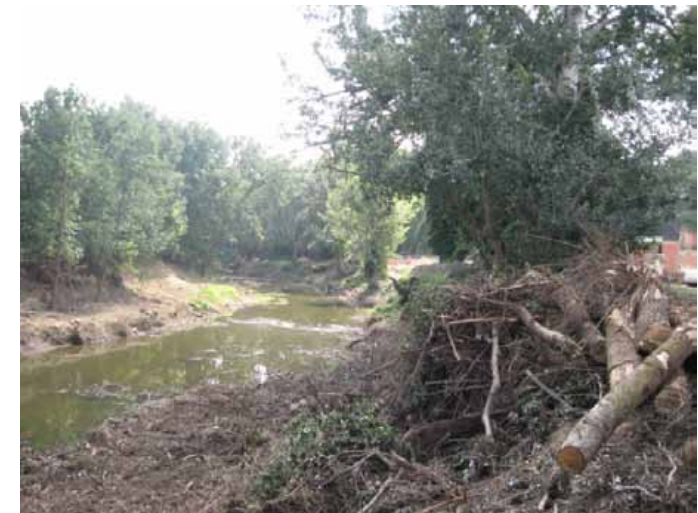
Creswick Creek being cleaned up following flood damage in Clunes- opportunity exists to reinstate and improve Creek Trail.
