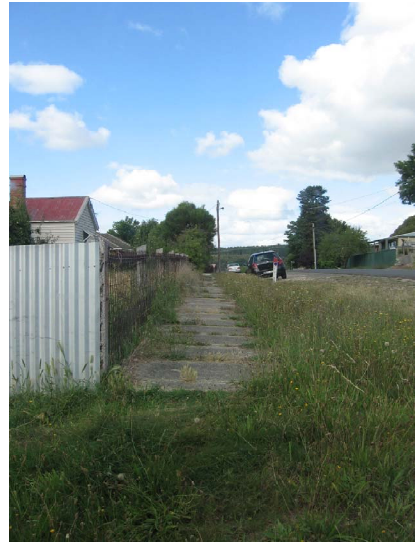
Hall Street Footpath, Creswick. Maintenance required.
